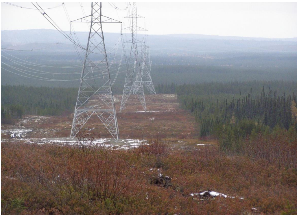
Figure 6 - Power line at Rose Site
